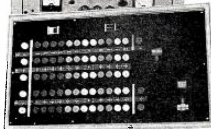
Typical Control Panel
